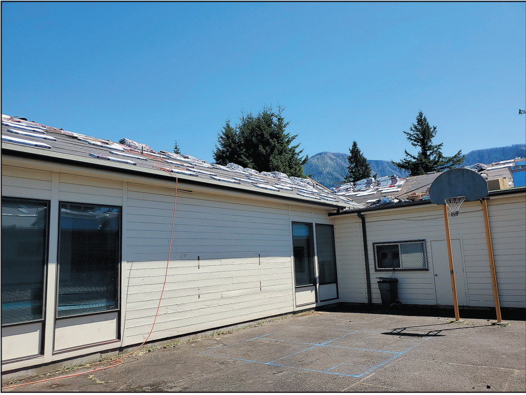
The renovation of Skamania School included replacing the courtyard roof. Photo provided by Skamania School
